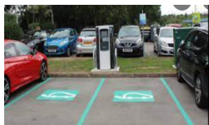
Communal EV charging points
